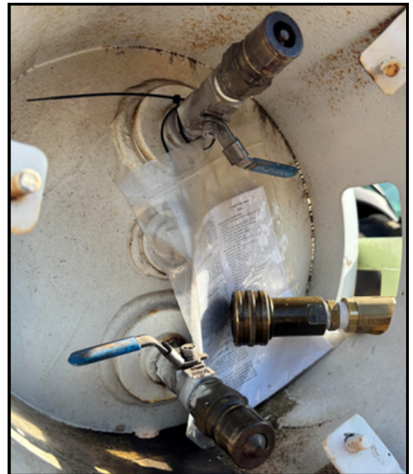
TOP QUICK CONNECT NOT SEATED PROPERLY UPON VISUAL INSPECTION
