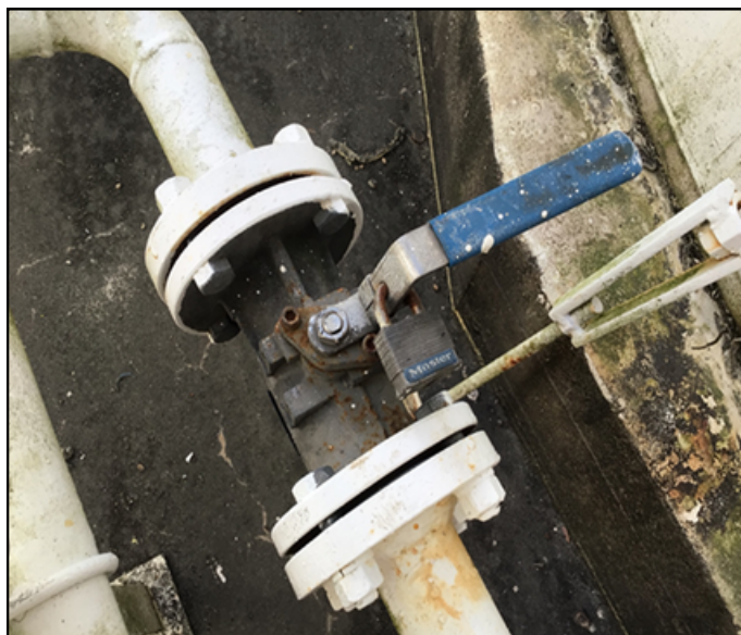
Padlock on valve in closed position when not in service.
