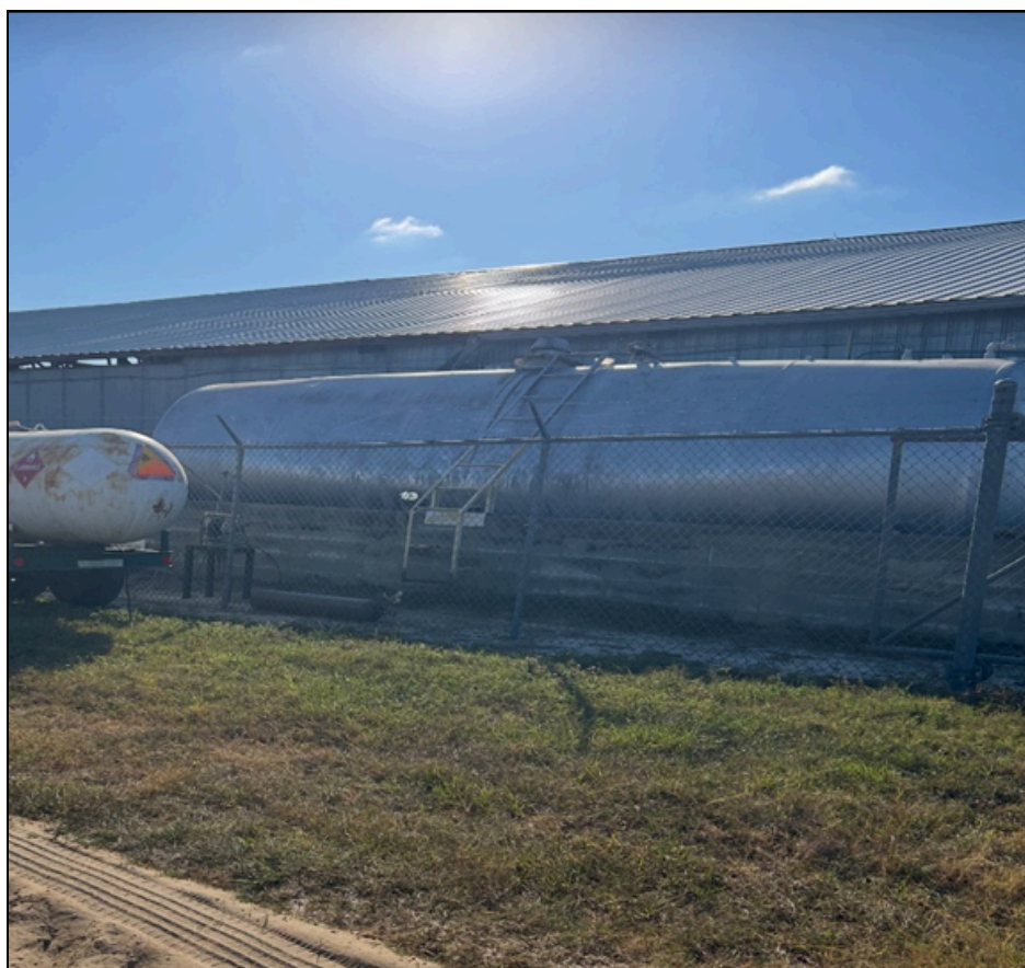
Security fencing around bulk tank.
